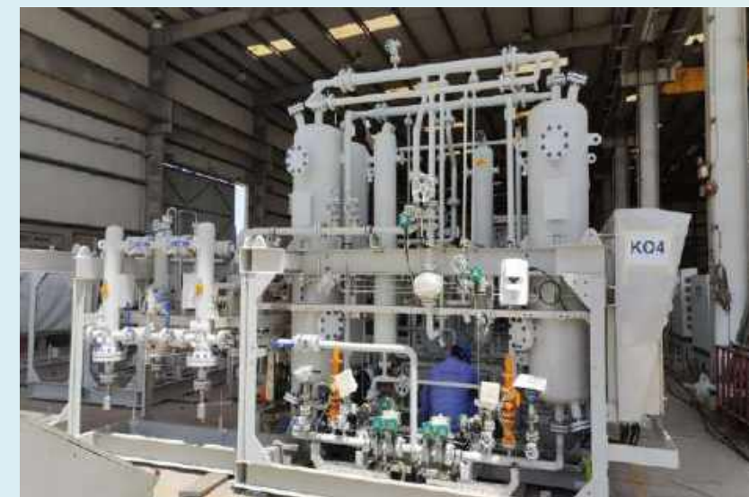
Air Dryer Skid
