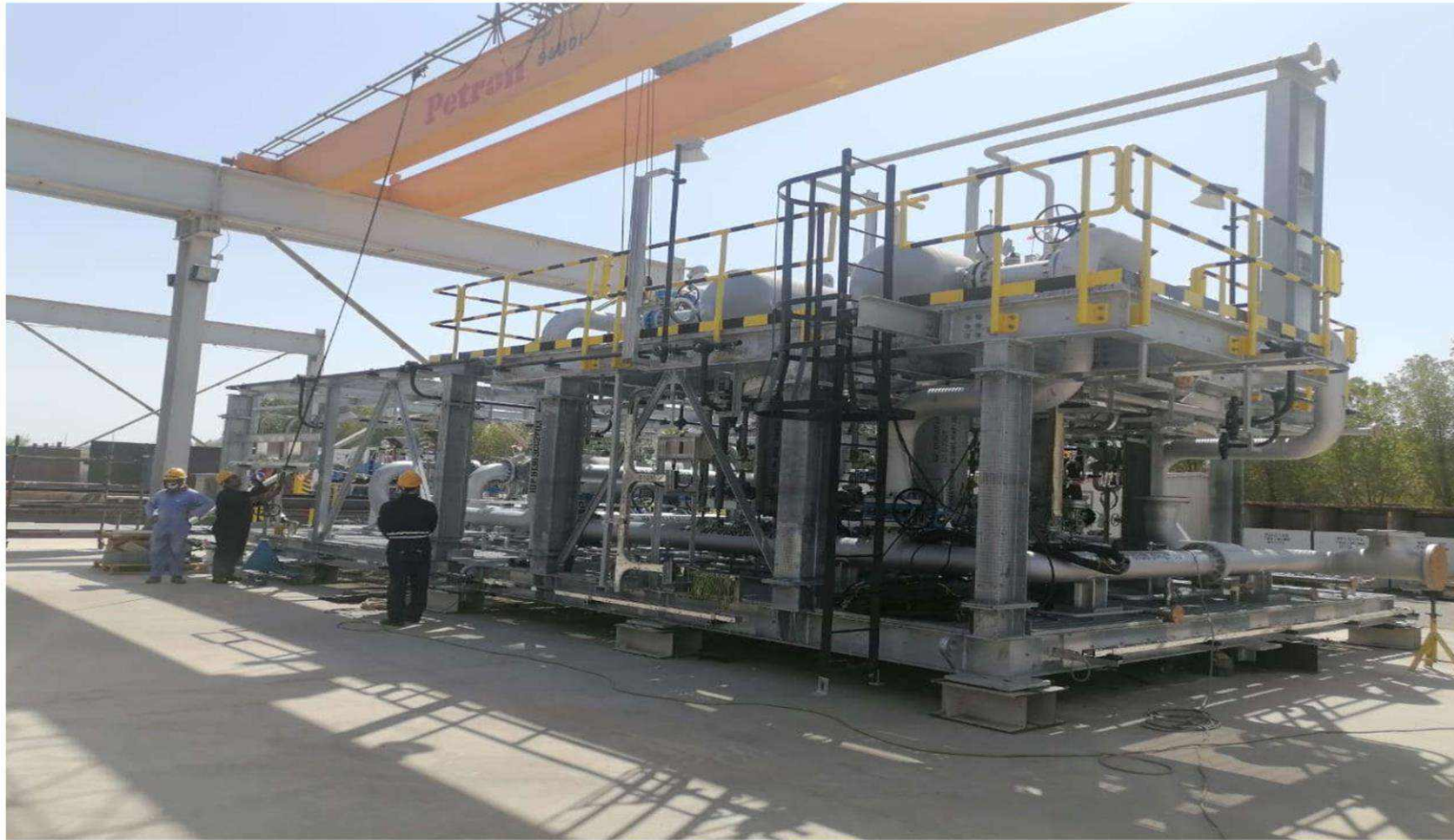
ARAMCO - SOUR CONDENSATE DEWATERING, KHURSANIYA PROJECT
